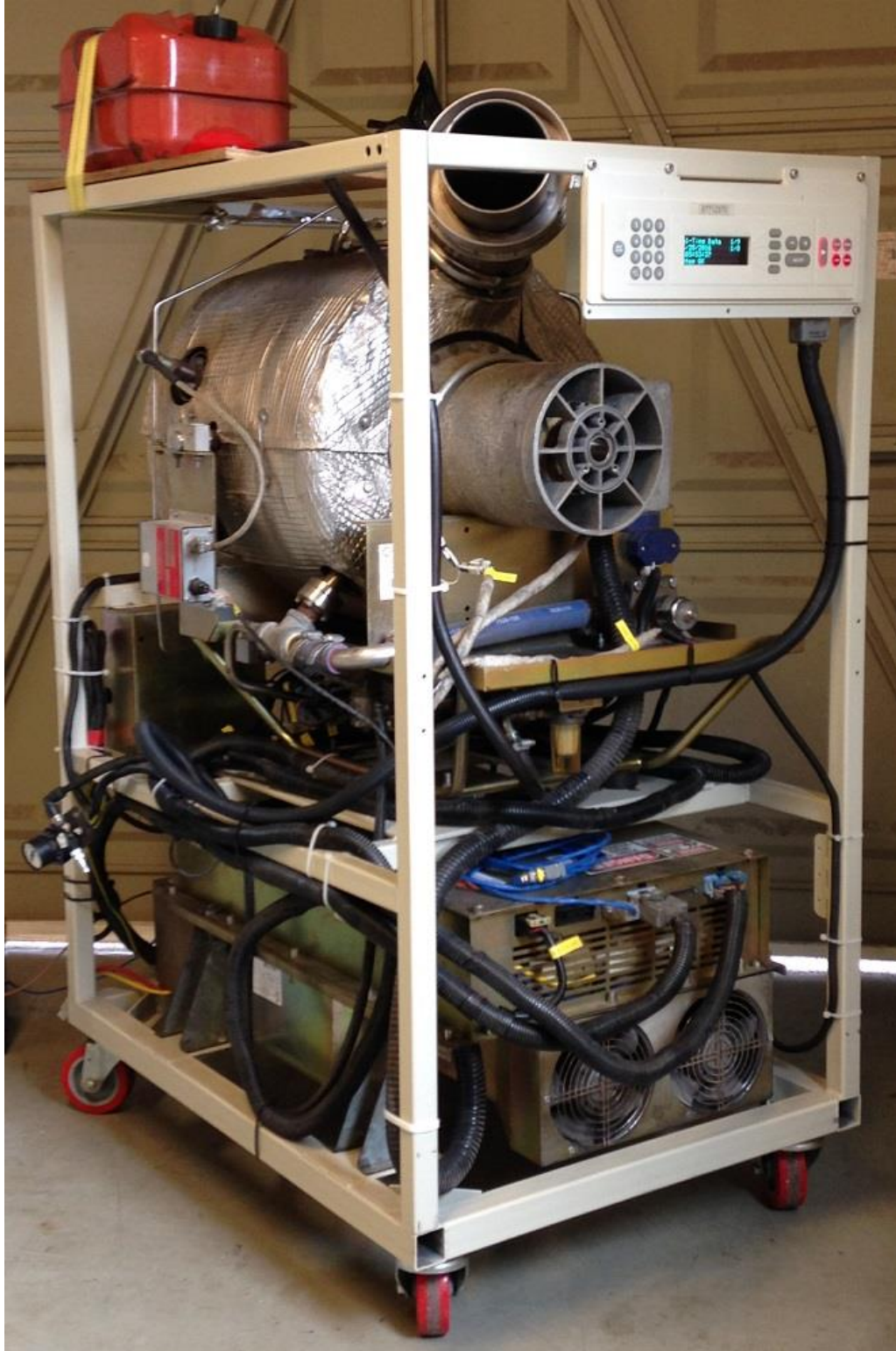
A 30KW Micro-turbine generator unit (Capstone C30)
