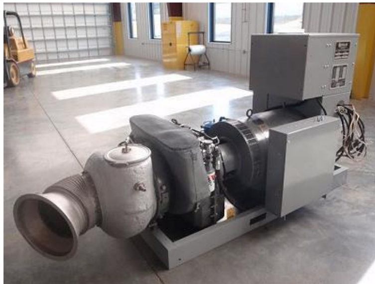
Solar Spartan GS350 300HP Gas Turbine
